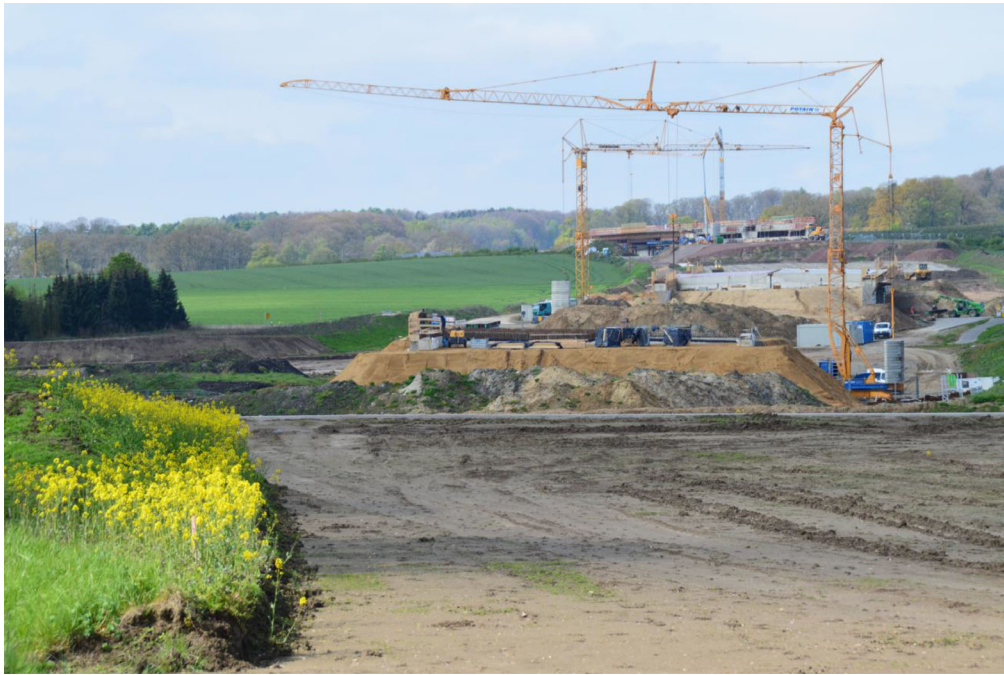
FIGURE 1 Extensive soil movements and construction activities for the ring road of the town Belm, near Osnabrück in 2017 (Photo: Maïke Bosold)
